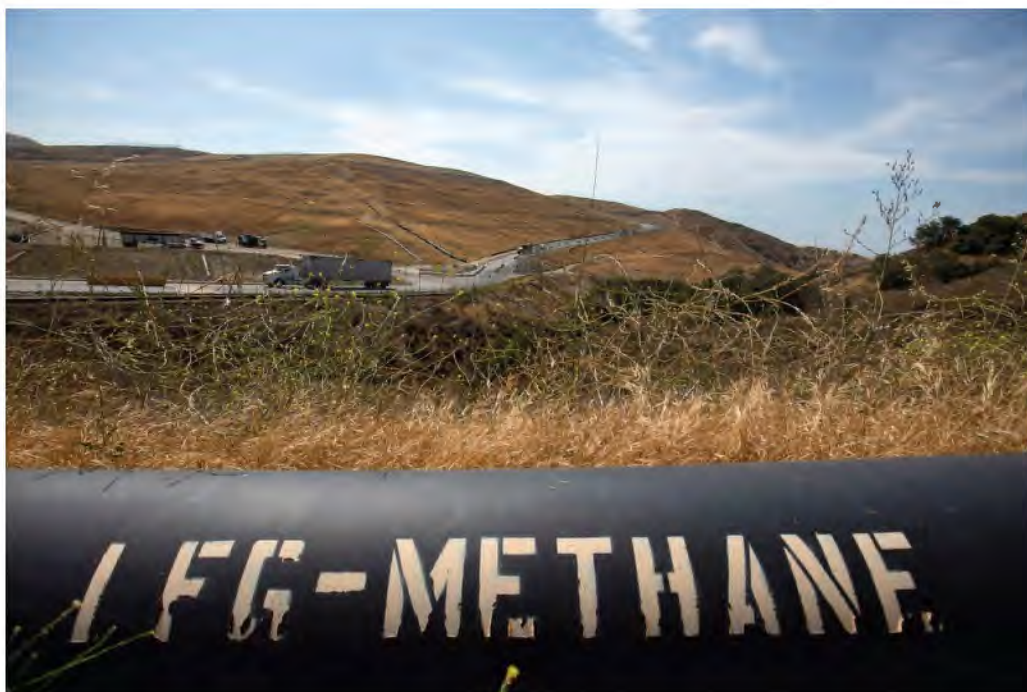
A pipeline that moves methane gas from the Frank R. Bowerman landfill to an onsite power plant is shown in Irvine, California, U.S., June 15, 2021. Picture taken June 15, 2021. REUTERS/Mike Blake/File Photo Purchase Licensing Rights
